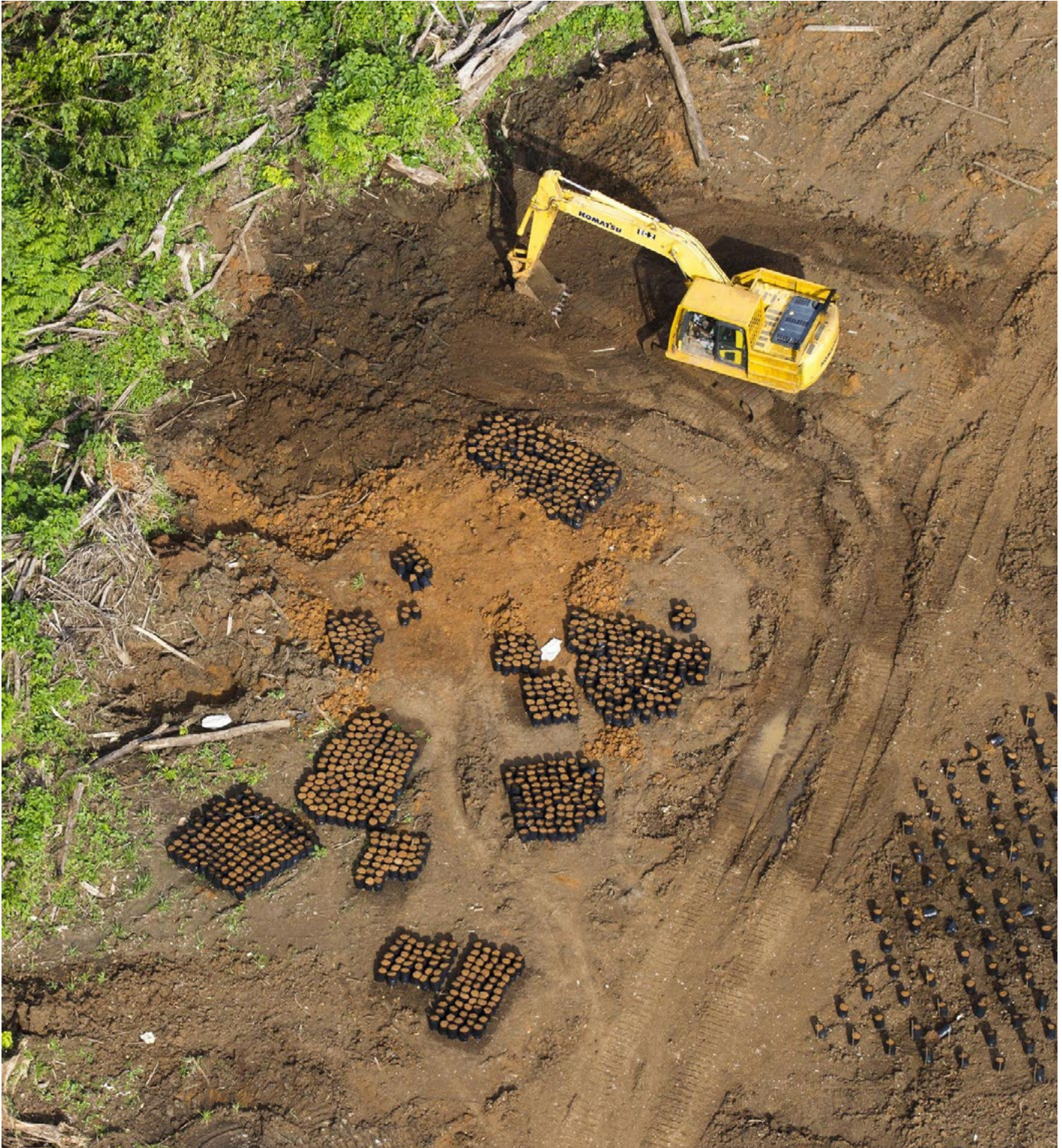
An excavator works the ground next to a palm oil nursery © Paul Hilton / Greenpeace
